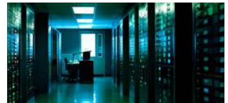
IN SERVER CENTERS
